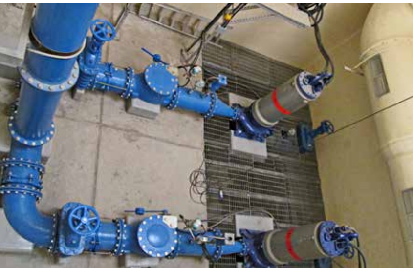
Pompstations, Abu Dhabi, VAE
